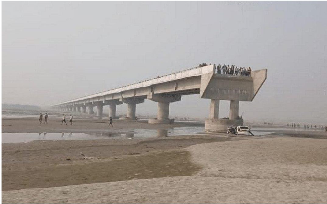
Fig 9. Bridge broke due to flood
