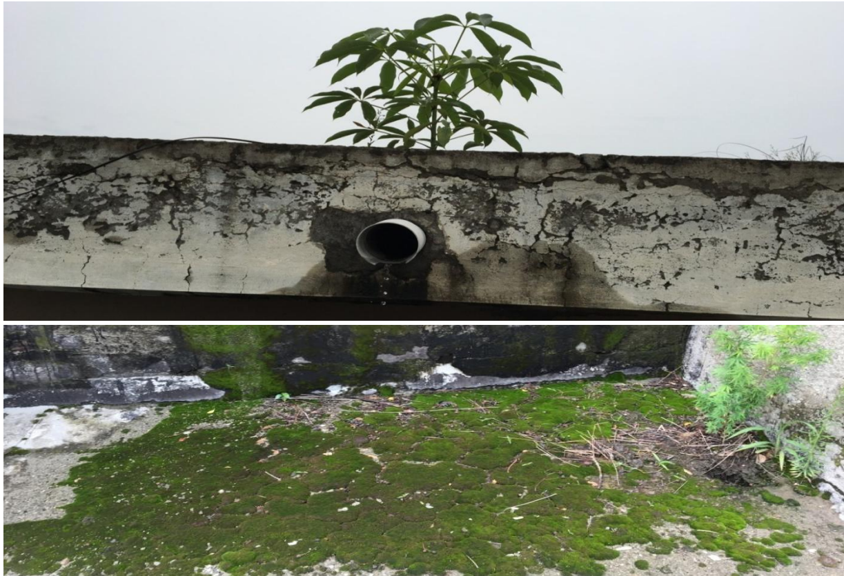
Fig.16 Biological growth Wild plant growth around building (Source: by Researcher)
