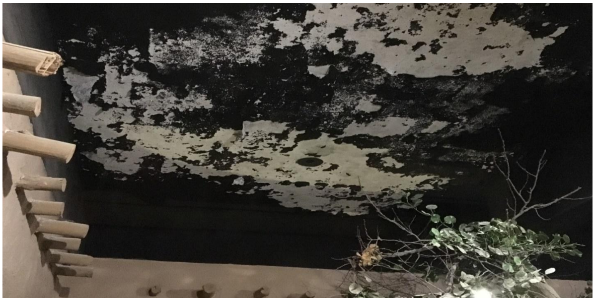
Fig.4 D-09 (ballads & romance): Efflorescence inside diorama due to RH & temp fluctuation on ceiling (Source: by Researcher)
